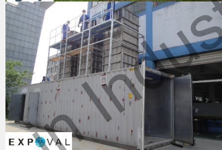
EXPOVAL Experimental plant on site 实验厂现场
